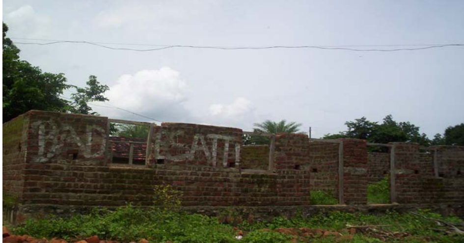
Picture 9: An incomplete school building in Badi Setty village, metres away from the overcrowded rooms in which students displaced from the ashram are staying.
